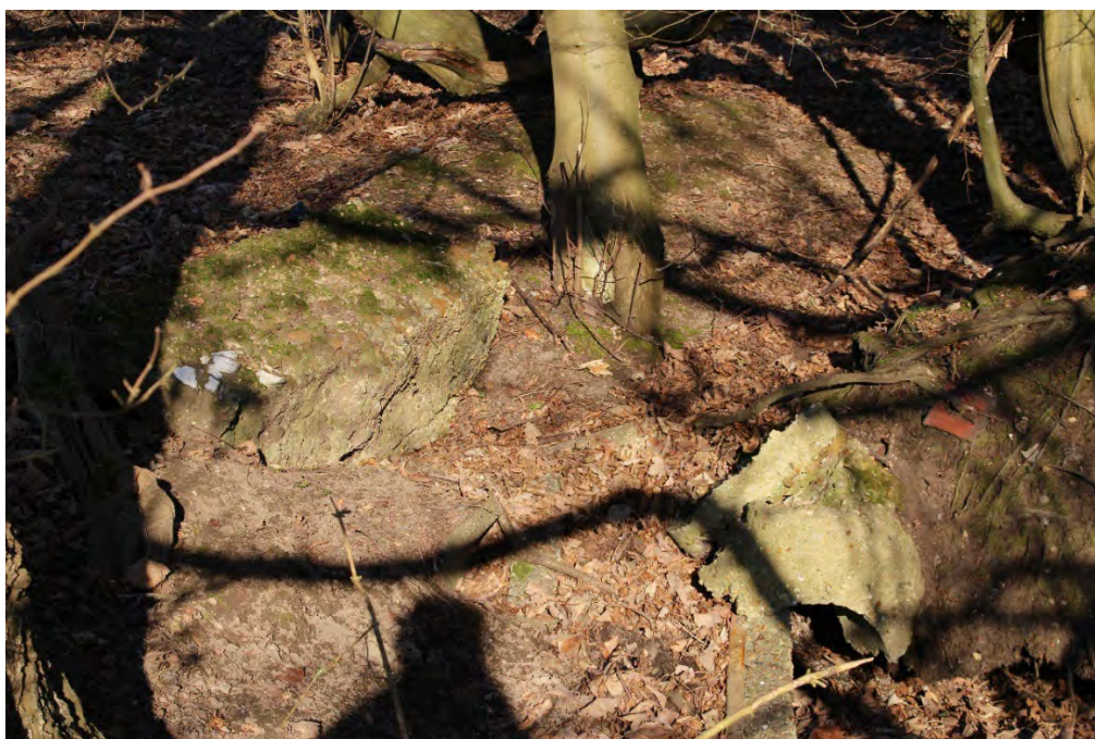
Figure 22 View 9, Concrete lying within northern part of pond, possibly drainage structure.
